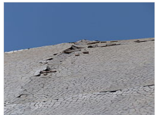
Missing and ill-fitting tiles on the wall of the Auditorio de Tenerife in 2015.
