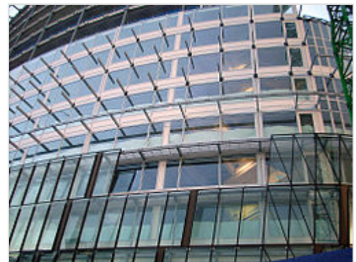
A Waagner-Biro double-skin facade being assembled at One Angel Square, Manchester . The brown outer facade can be seen being assembled to the inner white facade via struts. These struts create a walkway between both 'skins' for ventilation, solar shading and maintenance.
