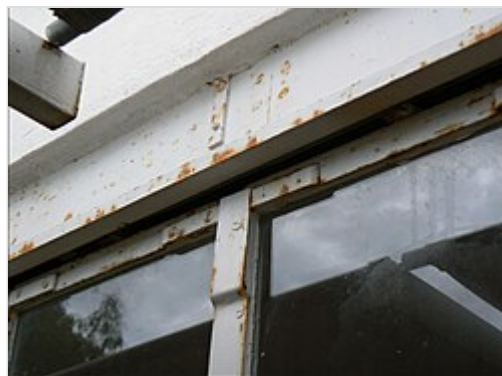
E-1027 after restoration (2013) corrosion of the frames and of the metal work
