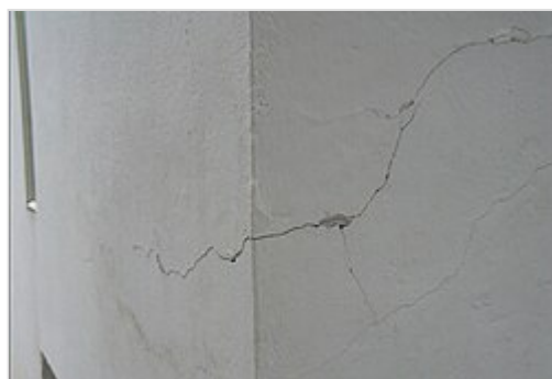
E-1027 after restoration (2013) one example of many cracked walls
